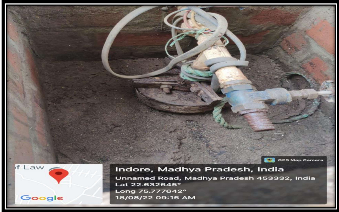
Bore Well No. 1
