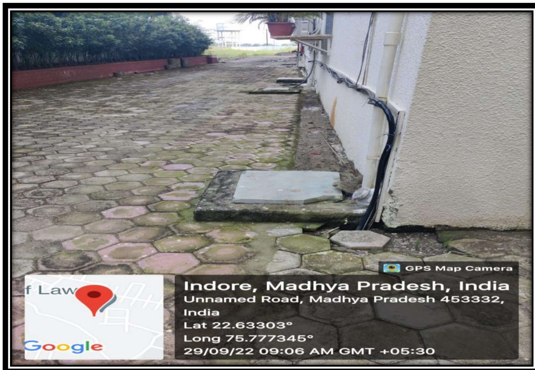
Chambers for Water distribution
