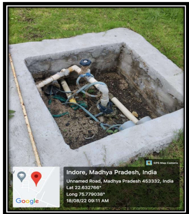
Bore Well No. 3
