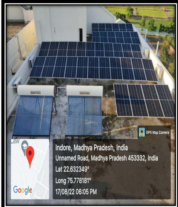
Solar Plant (Block – D)
