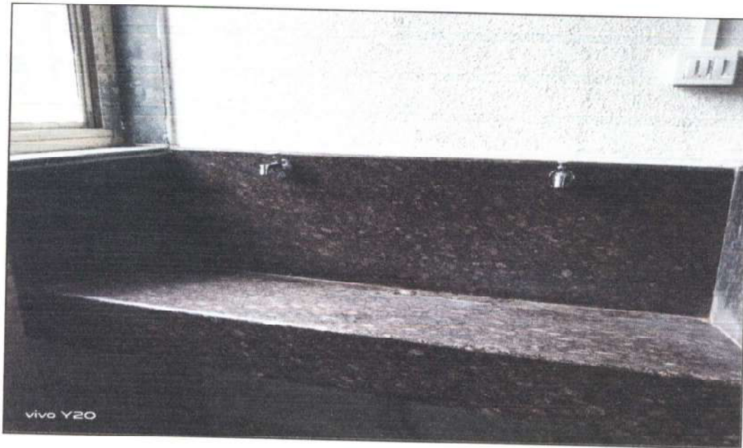
Figure: - 2.3 Water Taps
