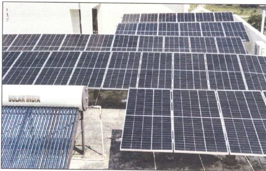
Figure 2.3:- Solar Plant 58 KWp and Inverter System
