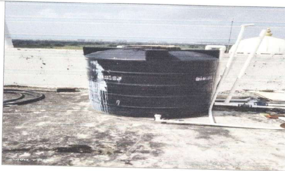
Fresh Water Storage tank
