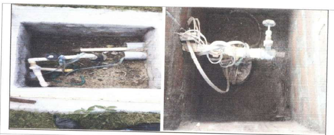
Figure2.1:-Fresh water source borewell
