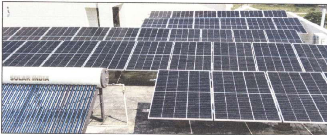
Figure 2.6:- Solar Plant 58 KWp and Inverter System
