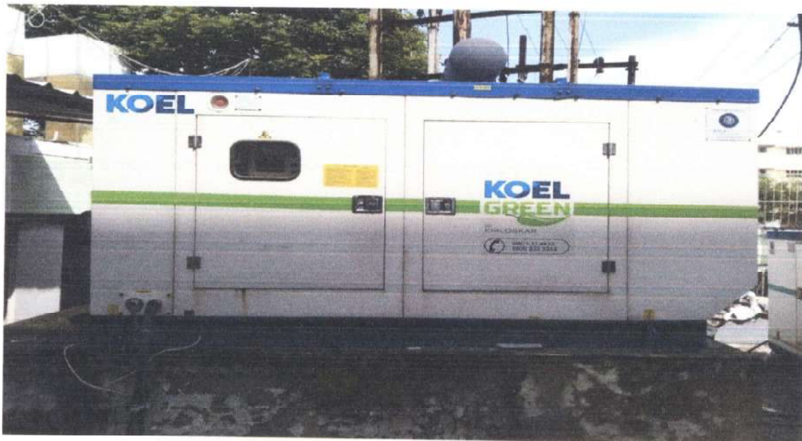
Figure 2.3:- DG set in power house
