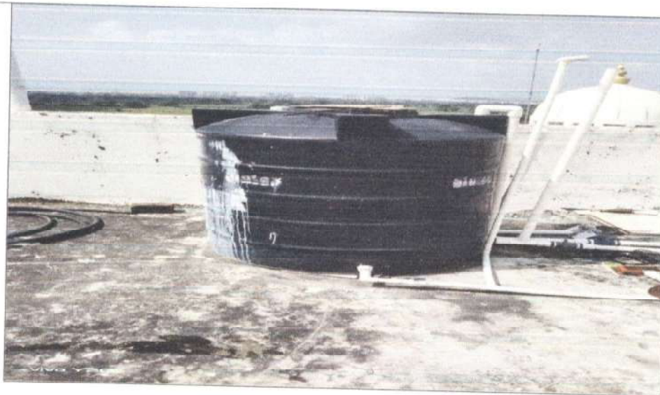
Fresh Water Storage tank
