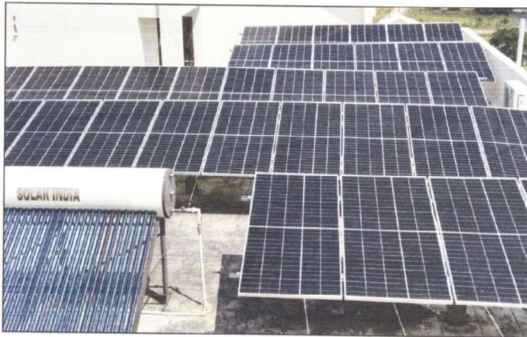
Figure 2.3:- Solar Plant 58 KWp and Inverter System
