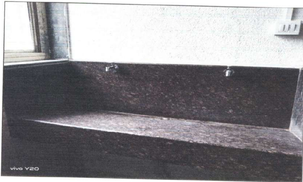
Figure: - 2.3 Water Taps
