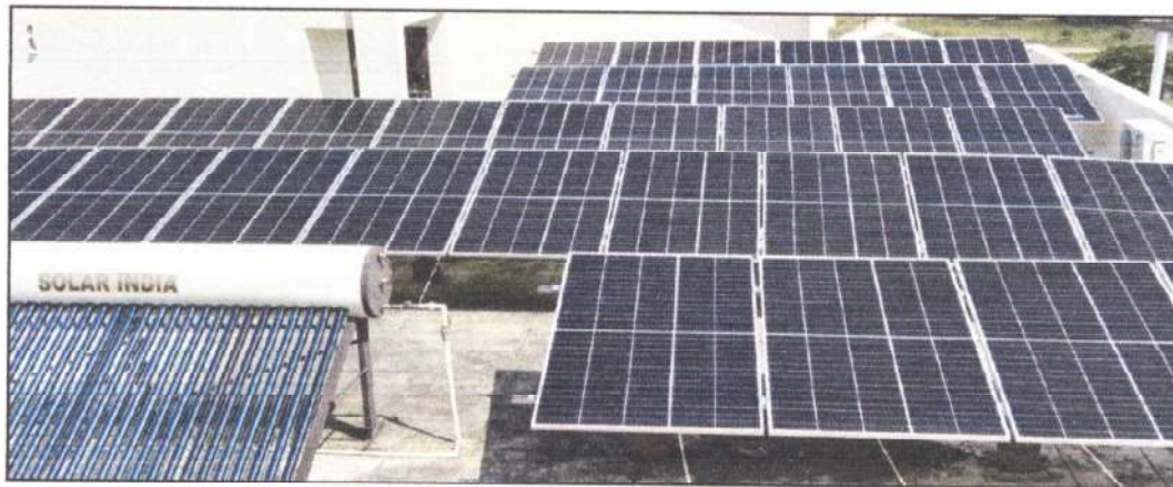
Figure 2.6:- Solar Plant 58 KWp and Inverter System
