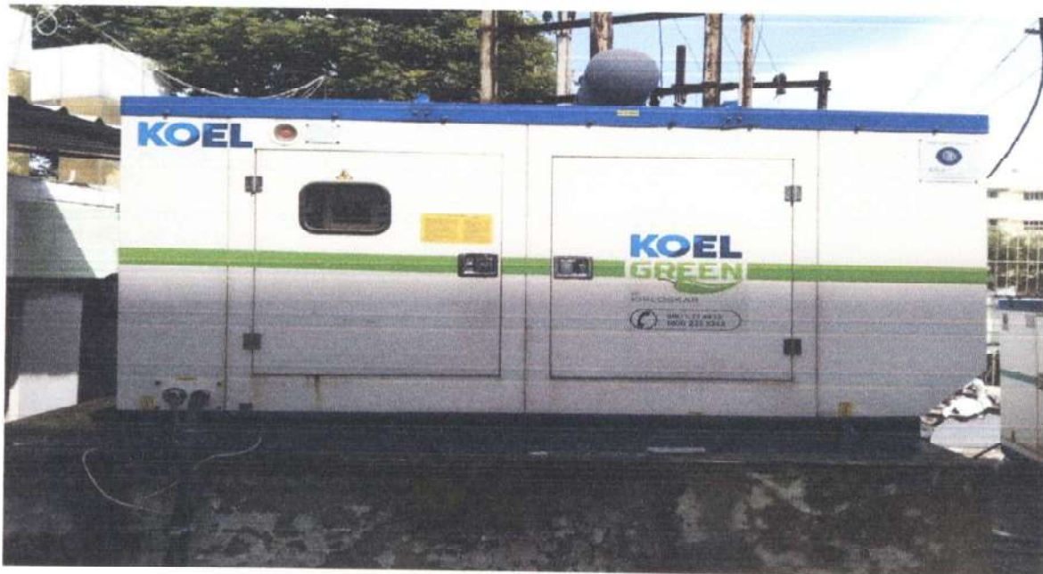
Figure 2.3:- DG set in power house
