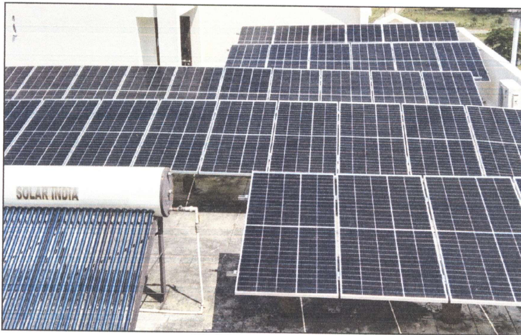
Figure 2.3:- Solar Plant 58 KWp and Inverter System
