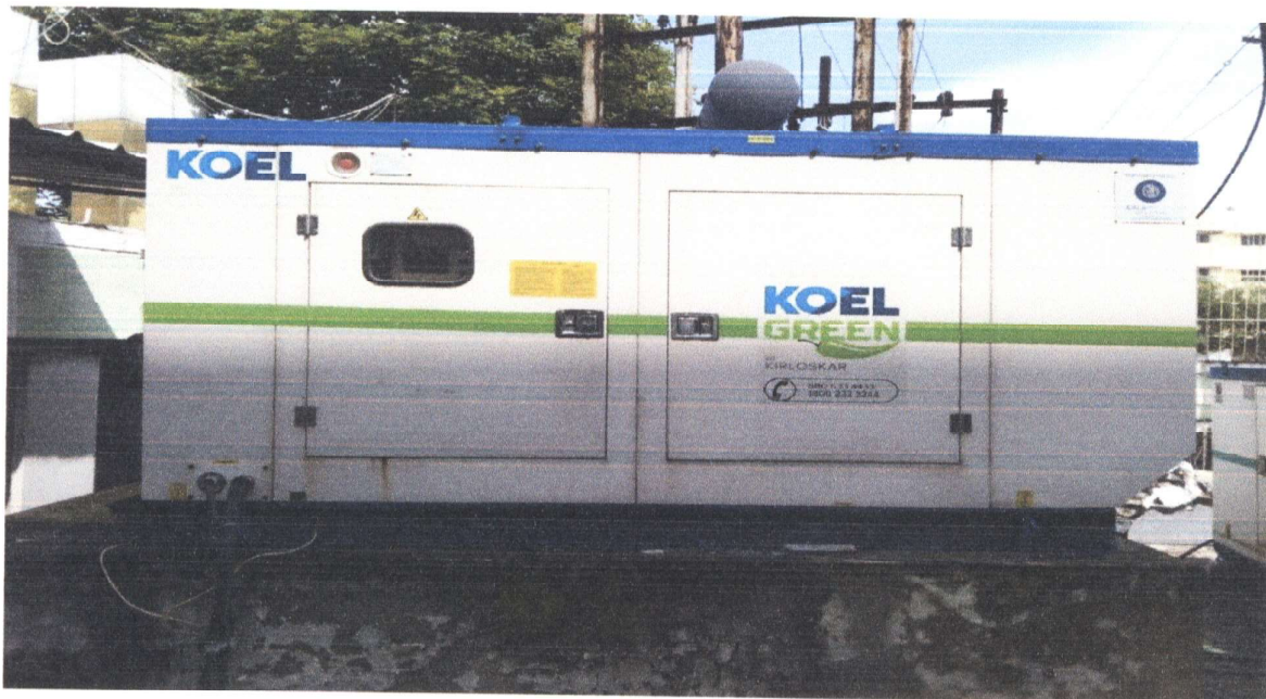
Figure 2.3:- DG set in power house
