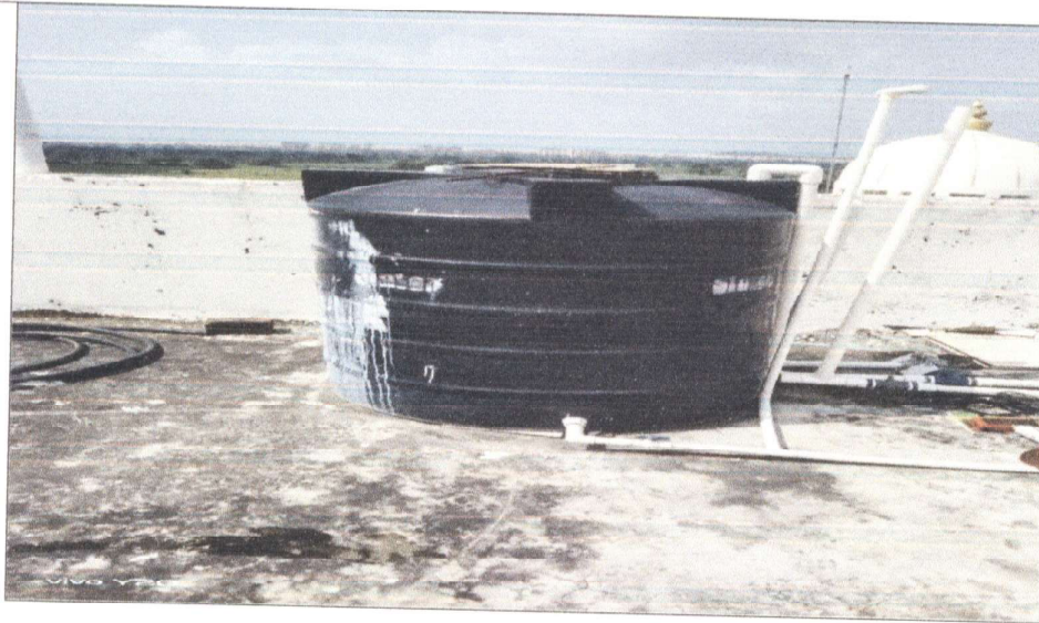
Fresh Water Storage tank
