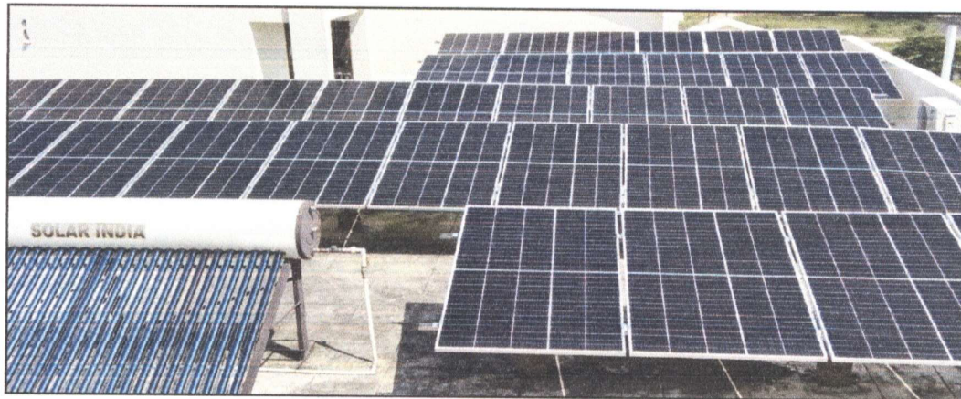
Figure 2.6:- Solar Plant 58 KWp and Inverter System
