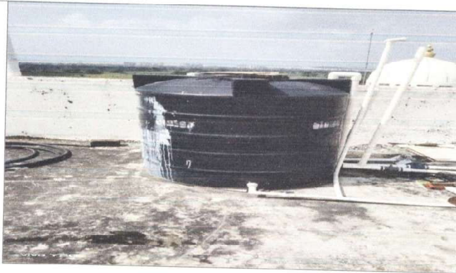
Fresh Water Storage tank
