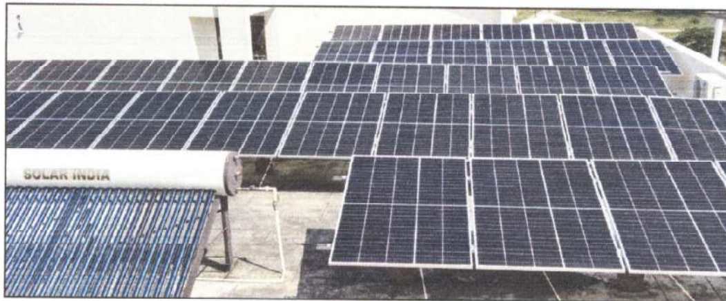
Figure 2.6.- Solar Plant 58 KWp and Inverter System
