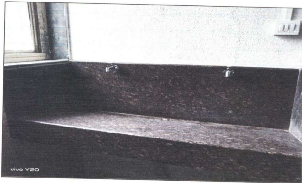
Figure: - 2.3 Water Taps
