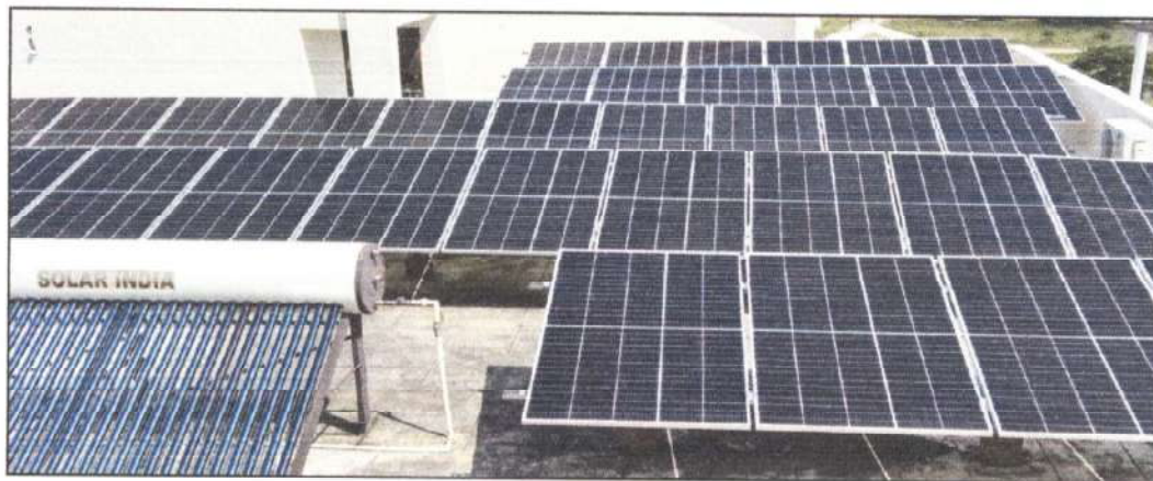
Figure 2.6.- Solar Plant 58 KWp and Inverter System
