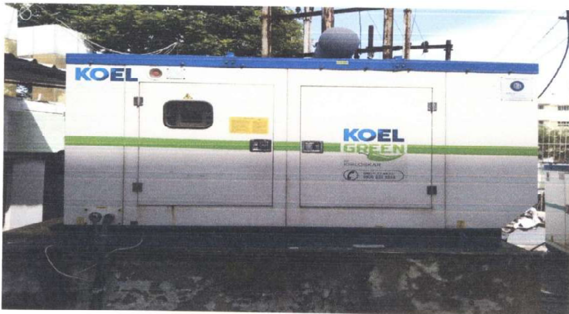
Figure 2.3:- DG set in power house
