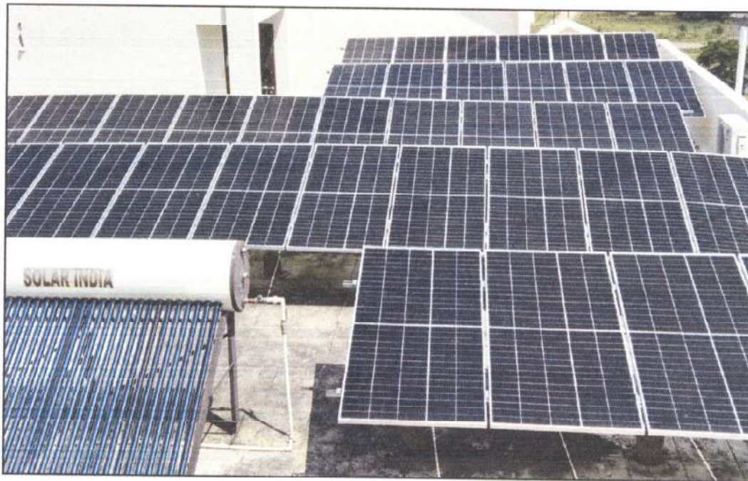
Figure 2.3:- Solar Plant 58 KWp and Inverter System
