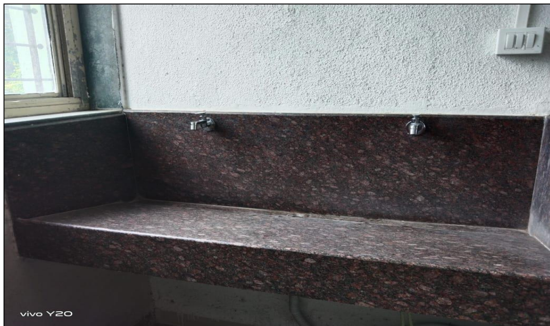
Figure:-2.3 Water Taps
