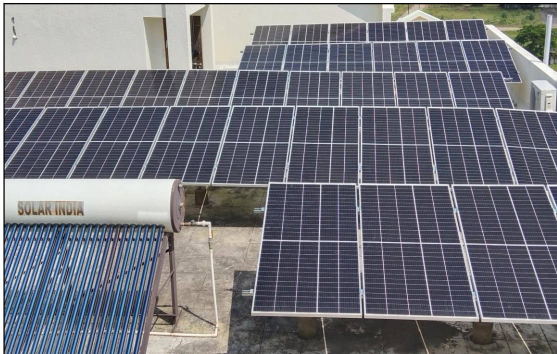
Photographs of Solar Plant:-
