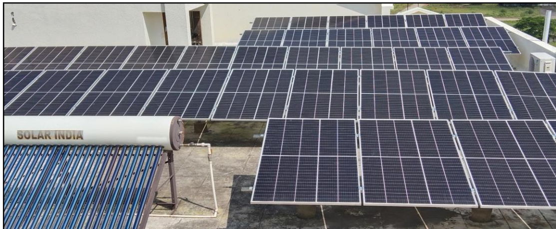
Photographs of Solar Plant:-
