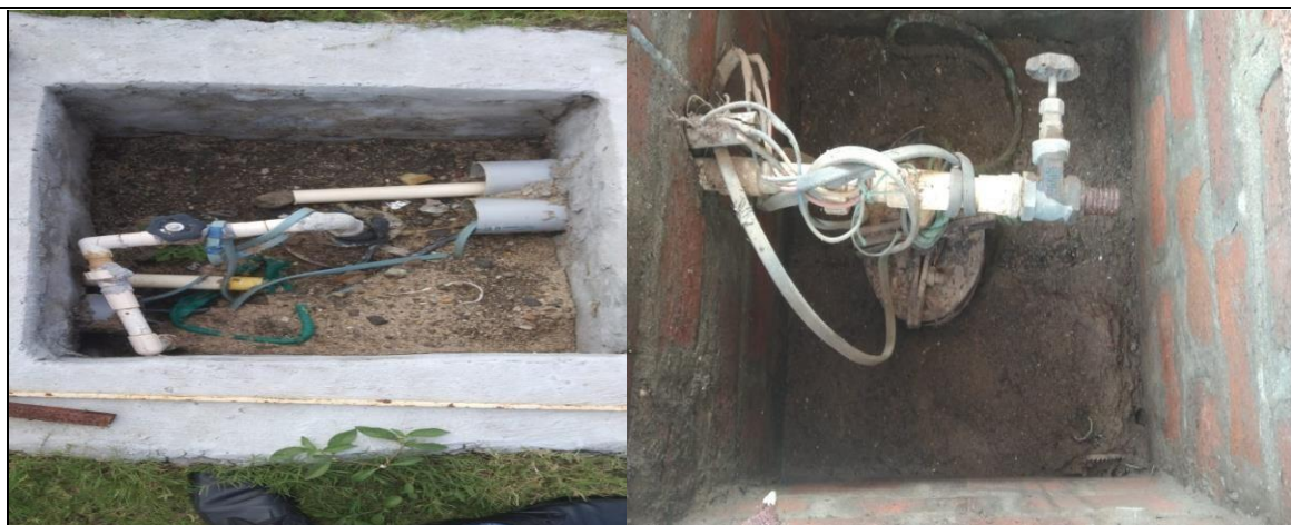
Figure 2.1:- Fresh water source bore well
