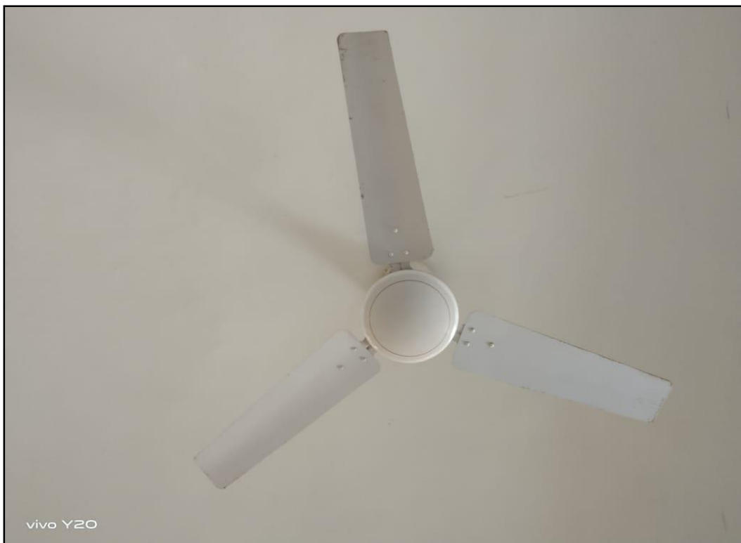
Figure 4.2:- Electrical Equipment in institute
