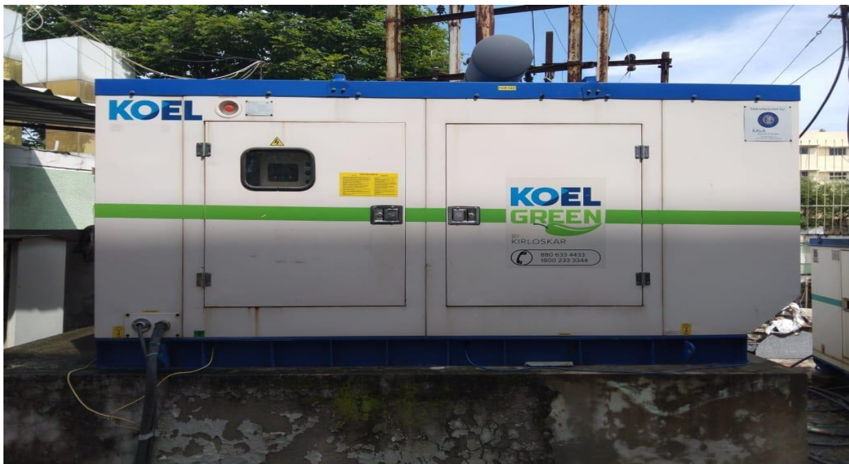
Figure 2.3:- DG set in power house
