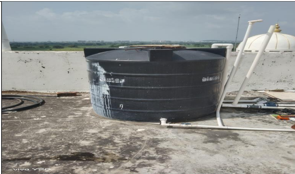
Fresh Water Storage tank
