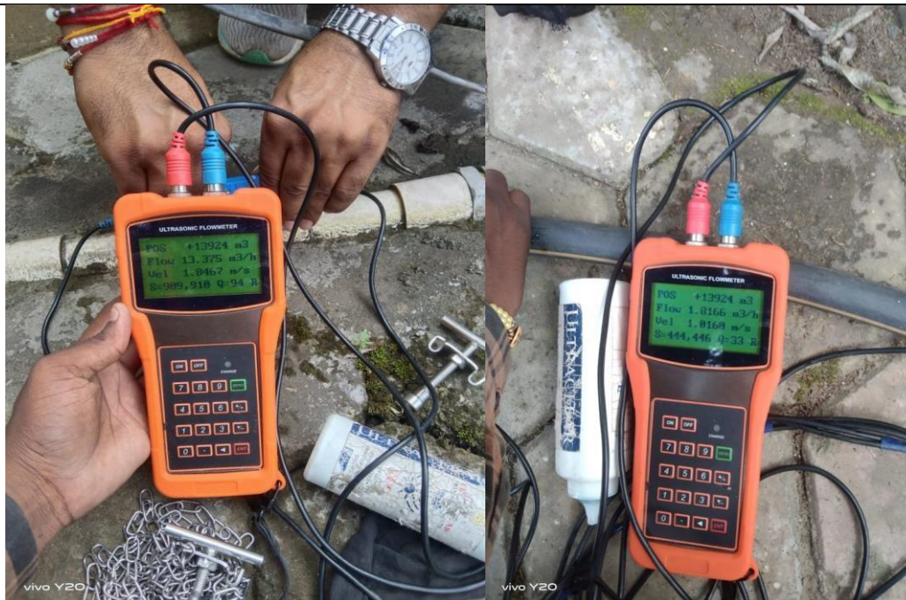
Ultrasonic flowmeter installation at institutetank
