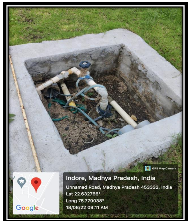
Bore Well No. 3
