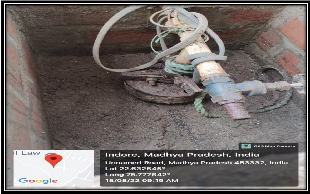
Bore Well No. 1
