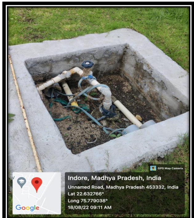
Bore Well No. 3
