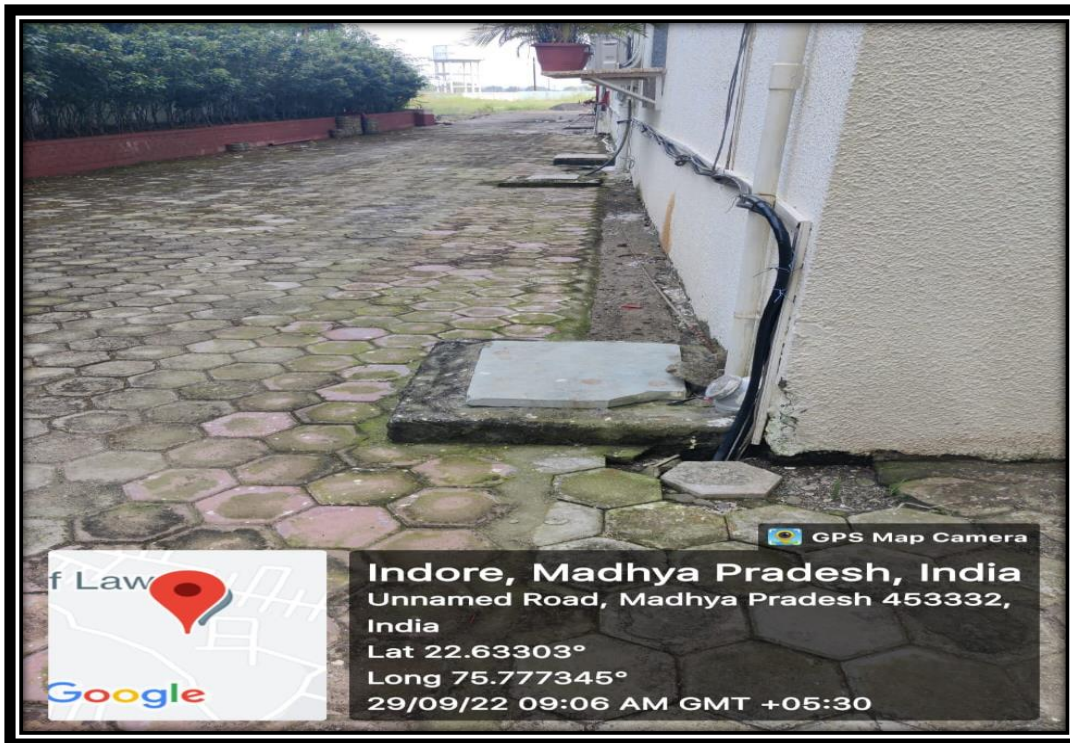
Chambers for Water distribution
