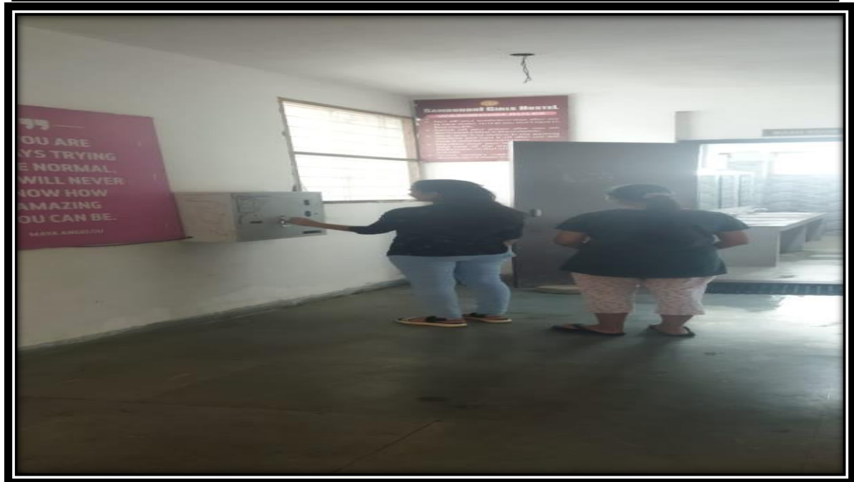
Sanitary Napkin Dispenser & Incinerator
