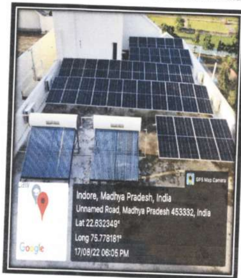
Solar Plant (Block – D)
